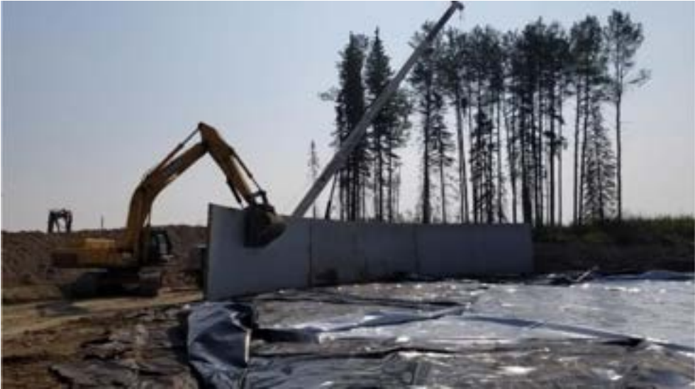
Temporary Water Storage Installation
